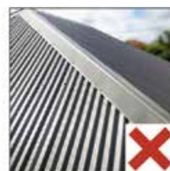
Unpainted metal work
