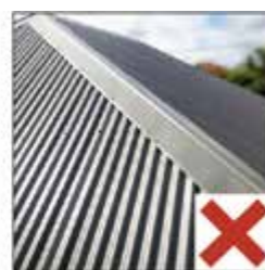
Unpainted metal work
